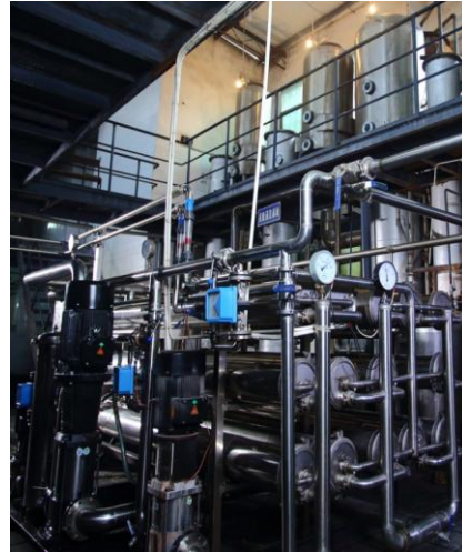
Filtration & Ion Exchange System
