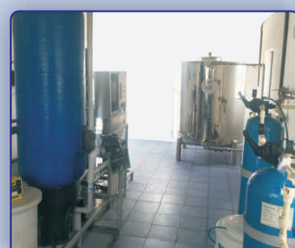
Purified Water Plant
