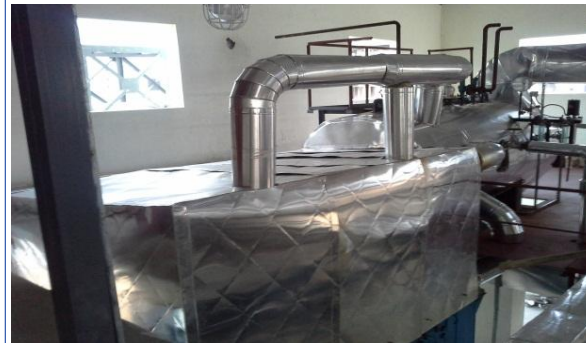
Boiler Equipment View
