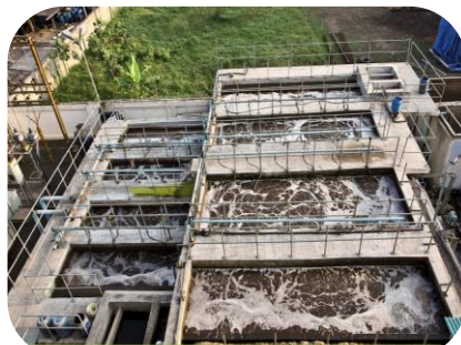
Effluent Treatment Plant
