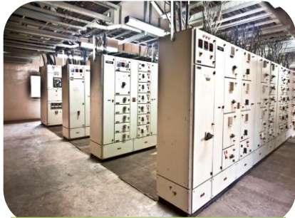
Electric Panel Room
