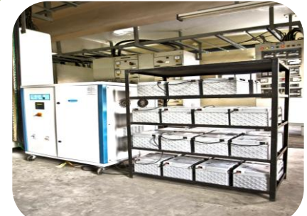
Uninterrupted Power Supply
