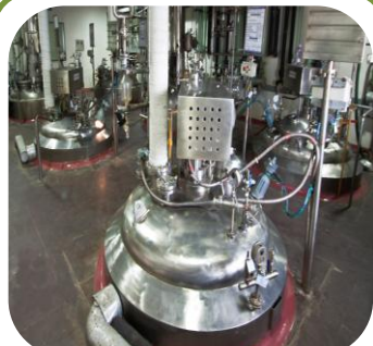
Glass Line Reactors
