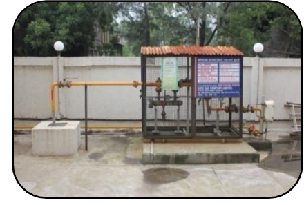
GSPC Gas Line
