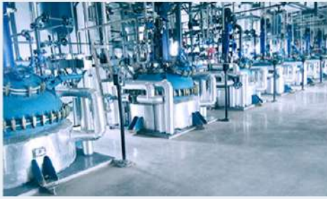
Chenghui Shuangda Pharmaceutical Industry — Workshop Equipment
