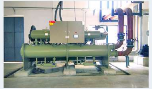
Chenghui Shuangda Pharmaceutical Industry — Air Conditioning Refrigerator
