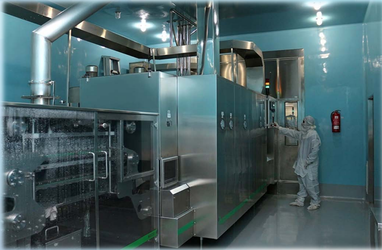
Vial Sterilizing tunnel
