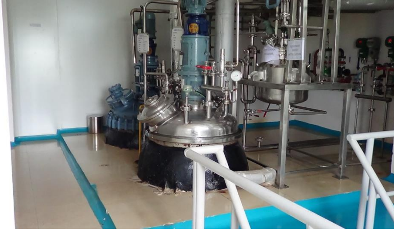
Purification Area (Mezzanine floor)
