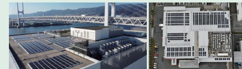
Solar panels installed on the roofs of Kewpie Kobe Plant (left) and Kitakami Delica Co., Ltd. (right).
