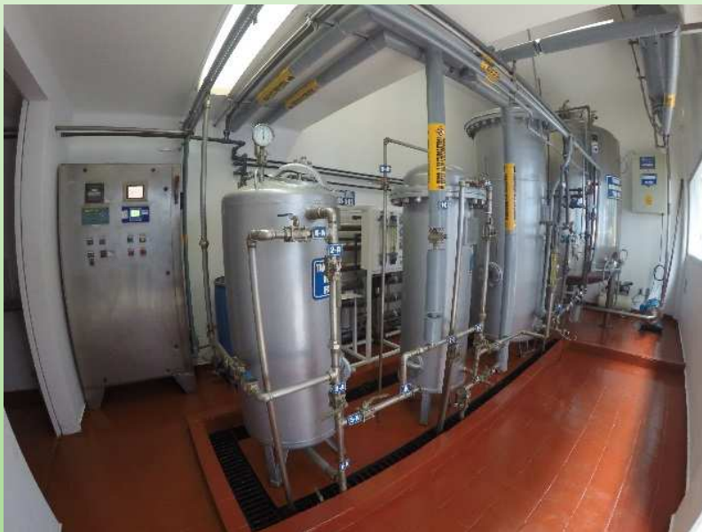
PW production plant
