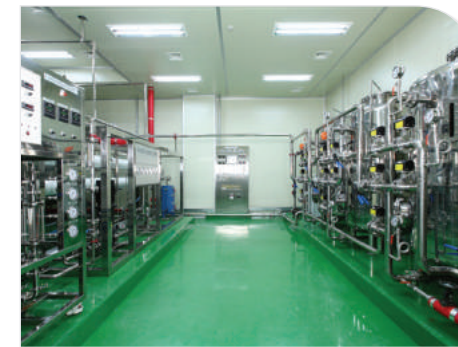
▶ Purified Water System
