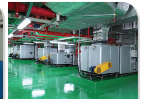
▶ Air Handling Unit
