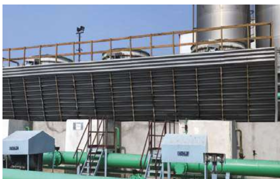
Cooling tower at the Toansa manufacturing site
