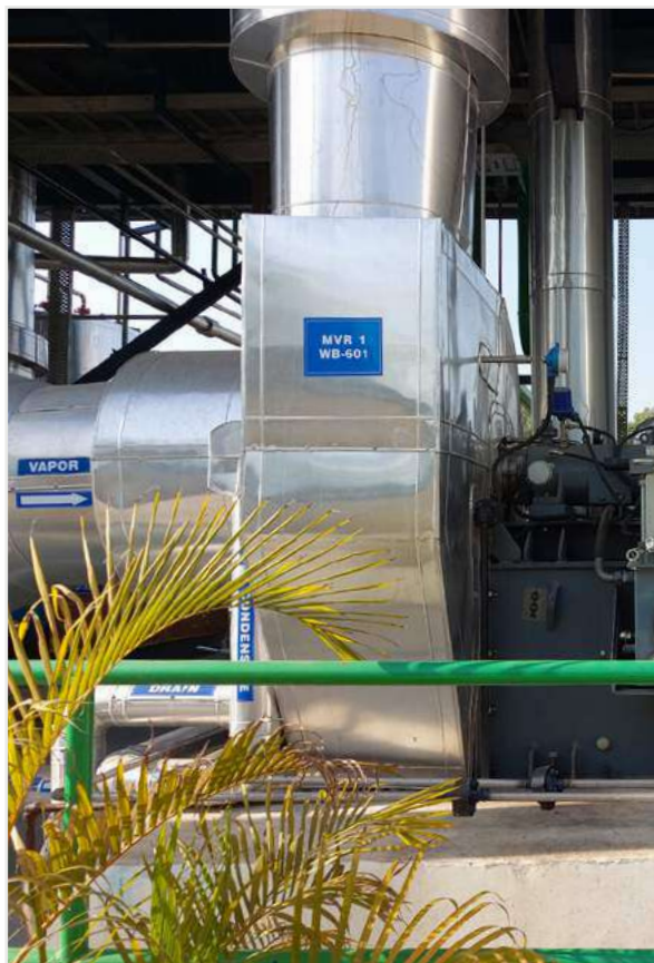
New MVR installation at Toansa wastewater treatment plant
