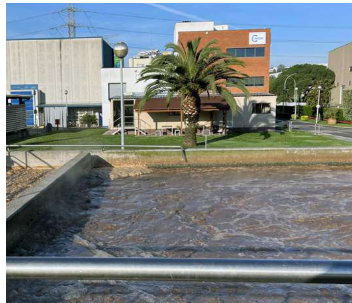
Part of the wastewater treatment facility installed in Spain
