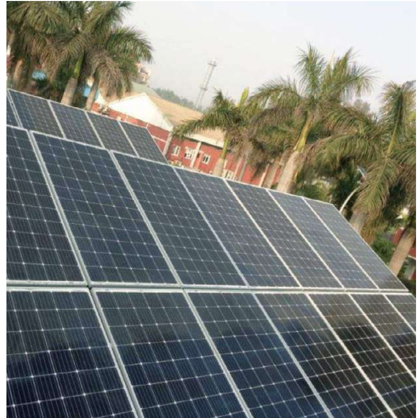
Roof-mounted solar panels on the administration office at Toansa
