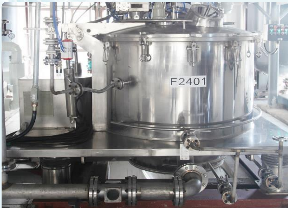
Reactor to Centrifuge
